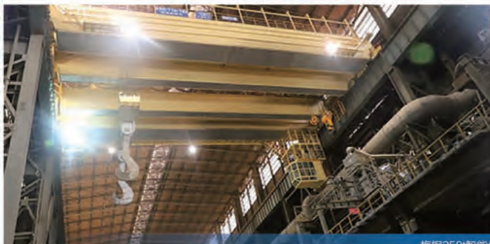
梅钢250t智能化铸造起重机 250t teeming crane used by Meishan Iron and Steel Co.,Ltd
