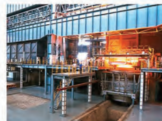
120t LF+VD 钢包精炼炉 120t LF+VD Ladle Refining Furnace
